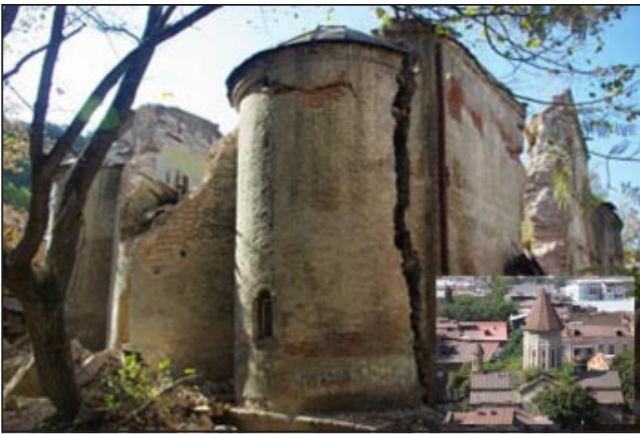
The collapsed section of Sourb Gevorg Church in Tbilisi (insert the church before the collapse)
